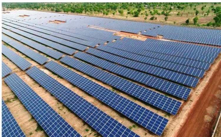
Fig. 1 Partial aerial view of the Zagtouli solar power plant
